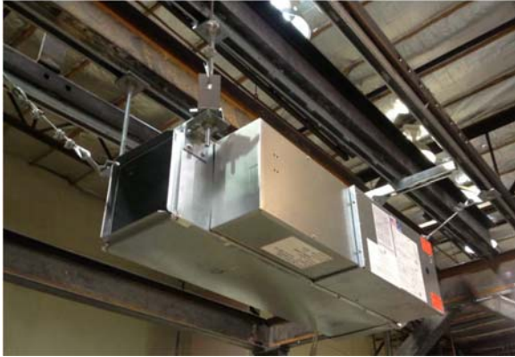
FIGURE 2 – SECTIONS OF 45-DEGREE AND 90-DEGREE BRACKETS WITH 3/8" or 1/2" DIAMETER ALL-THREADED ROD AND 3/16" DIAMETER STEEL CABLING ARE USED TO HANG THE VAV UNITS.
